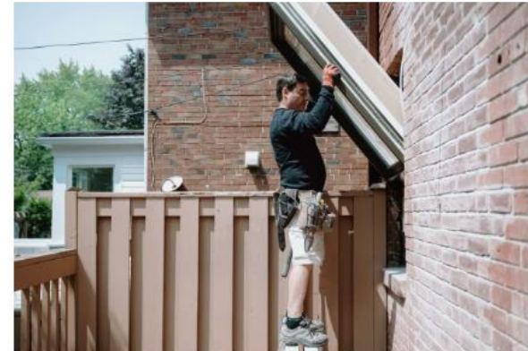
Domenic Masellis installs new windows in a house in Toronto on June 29. GALIT RODAN/THE GLOBE AND MAIL
